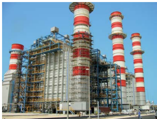
Siemens SGT5-4000 gas turbine in Qatar.
