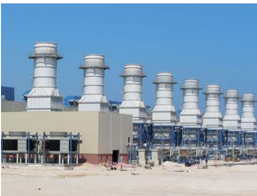
Siemens V 94.2 gas turbine in Middle East.
